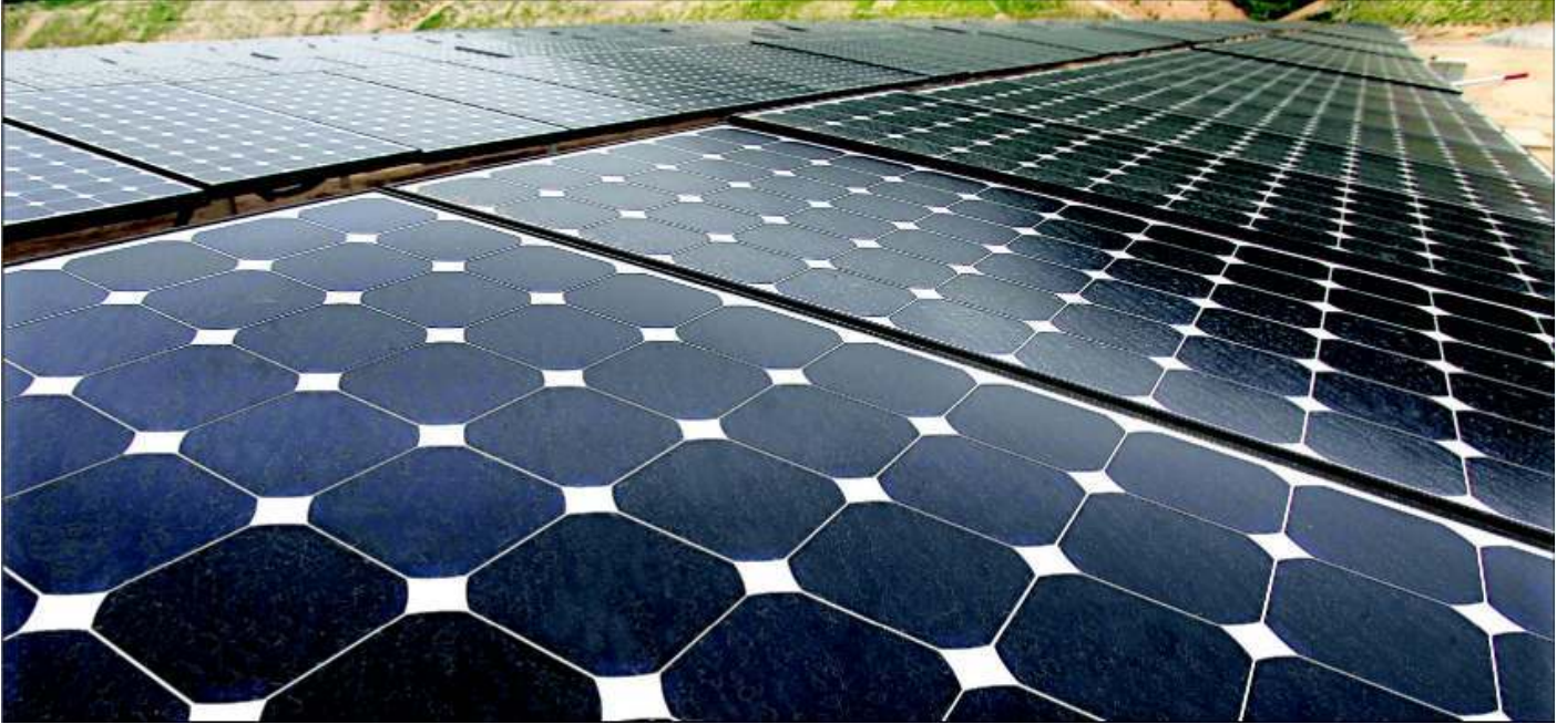
Expensive power: The cost of solar panels may be the big stumbling block for Pankaj Oswal's ambitious Pilbara power plans
