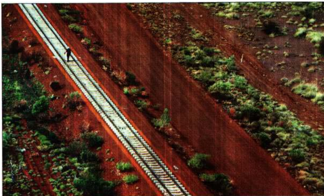
Fortescue says it needs to build the rail line because it has been denied access by BHP Billiton.
