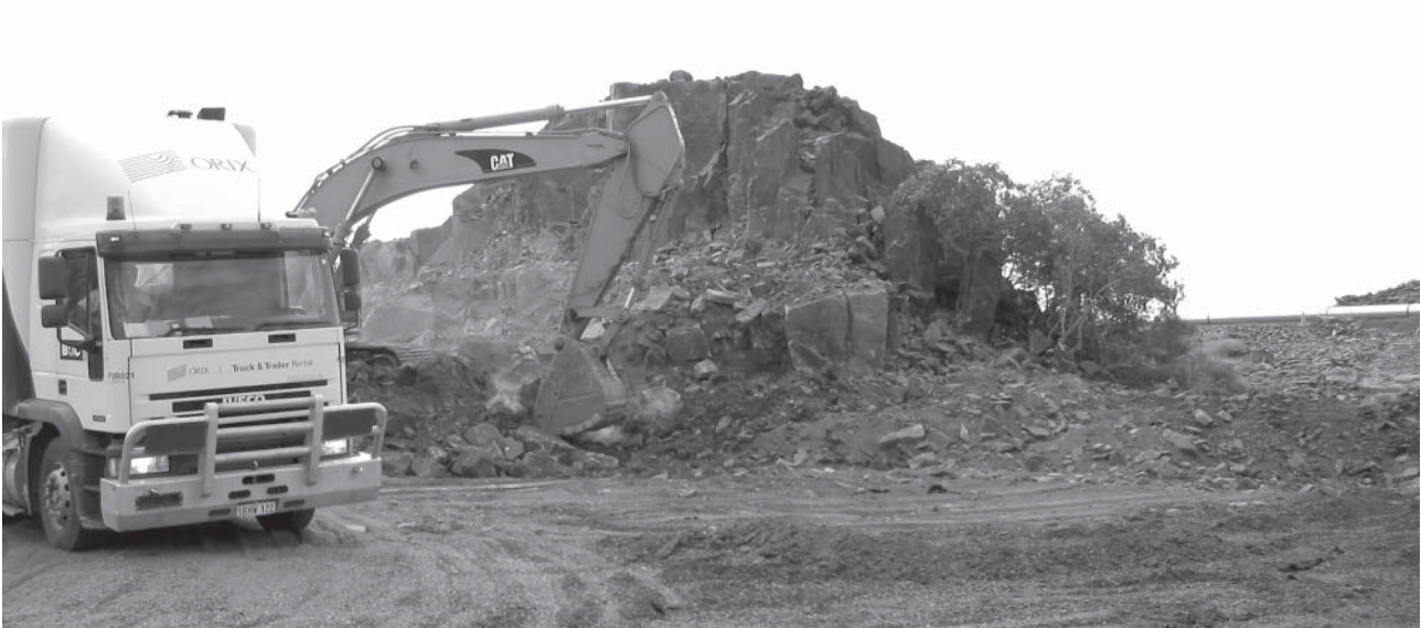
Figure 2. Destruction of rock art site for road fill, on 30 May 2006, near Dampier Port.
